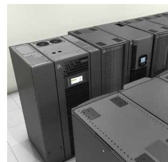
Liebert eXM adjacent to the wall
